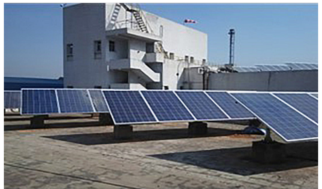
Figure 3. Solar Grid, Mother Dairy, Patparganj Unit, Delhi (India).
